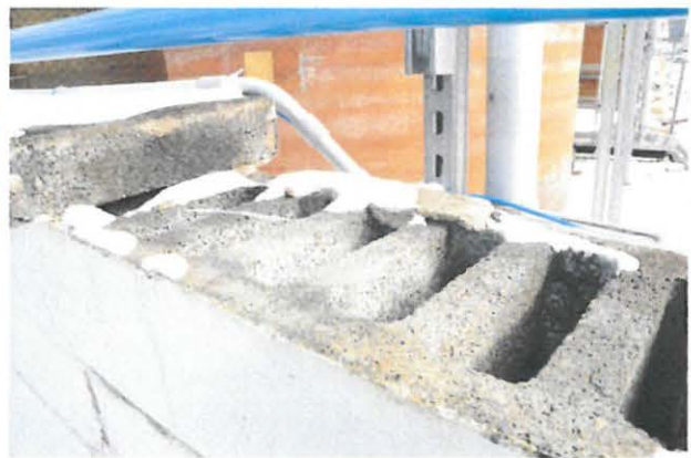
Missing cap on containment wall facing Elk River
